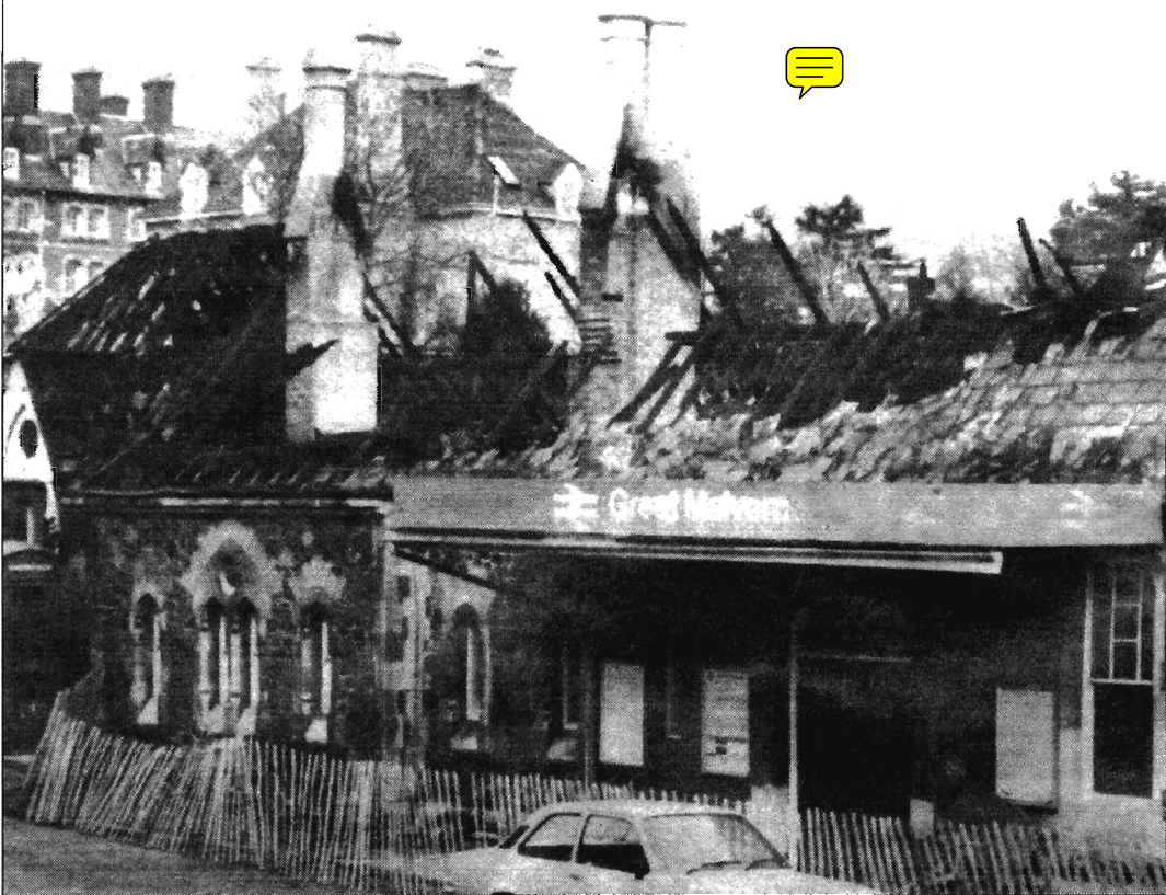
▲ THIS was the sad state of Great Malvern railway station 25 years ago after a fire seriously damaged the 125-year-old listed building. The blaze was particularly ill-timed, as a major renovation project at the station had just been completed. The roof was almost completely destroyed, and the tea room, waiting rooms, ticket office and toilets were badly damaged. However, British Rail promised to restore the station to its former glory.
